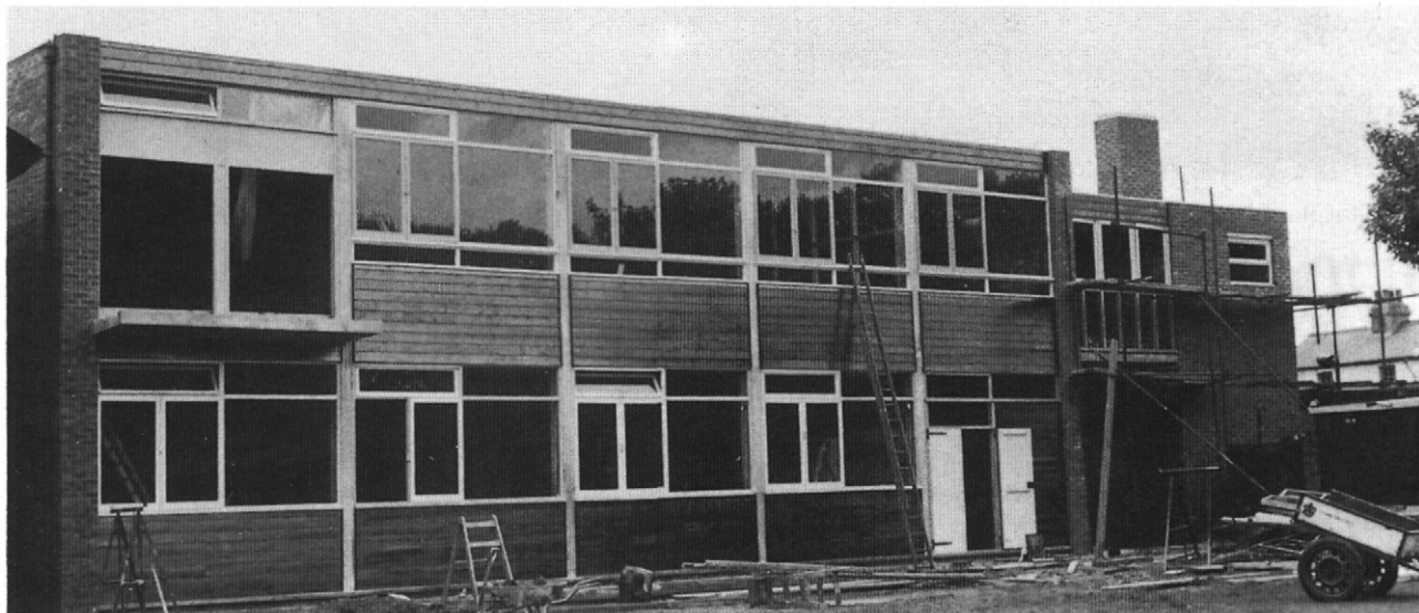
Art Room and Music Room: another part of the 1960s development — Art Room on the top, Music Room on the
